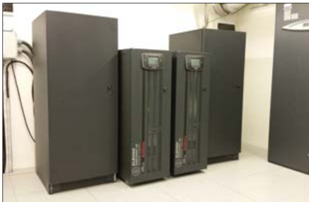
Datahall 2x40kVA parallell
