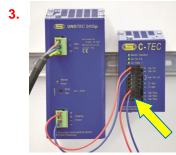
3. Connect the load to the buffered 24 V DC output of the C-TEC
